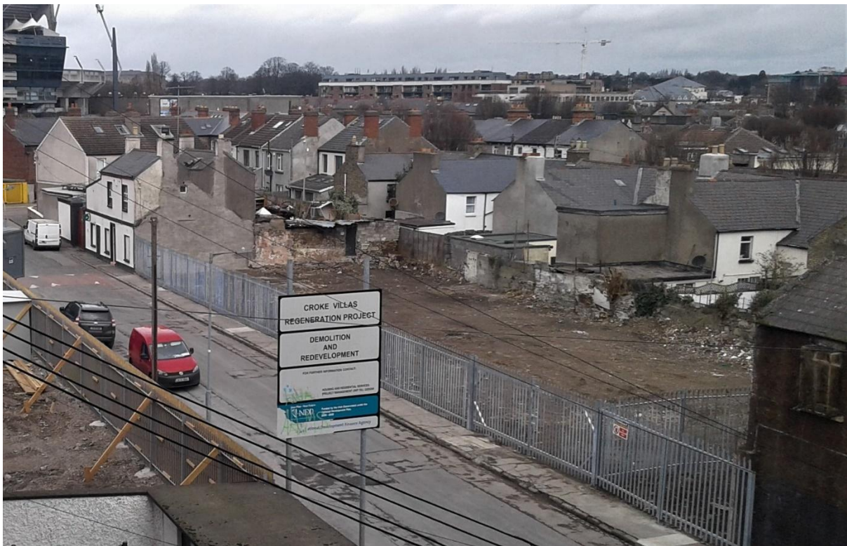
Demolition work on the former cottages on Sackville Avenue is now complete and the two sites cleared.
